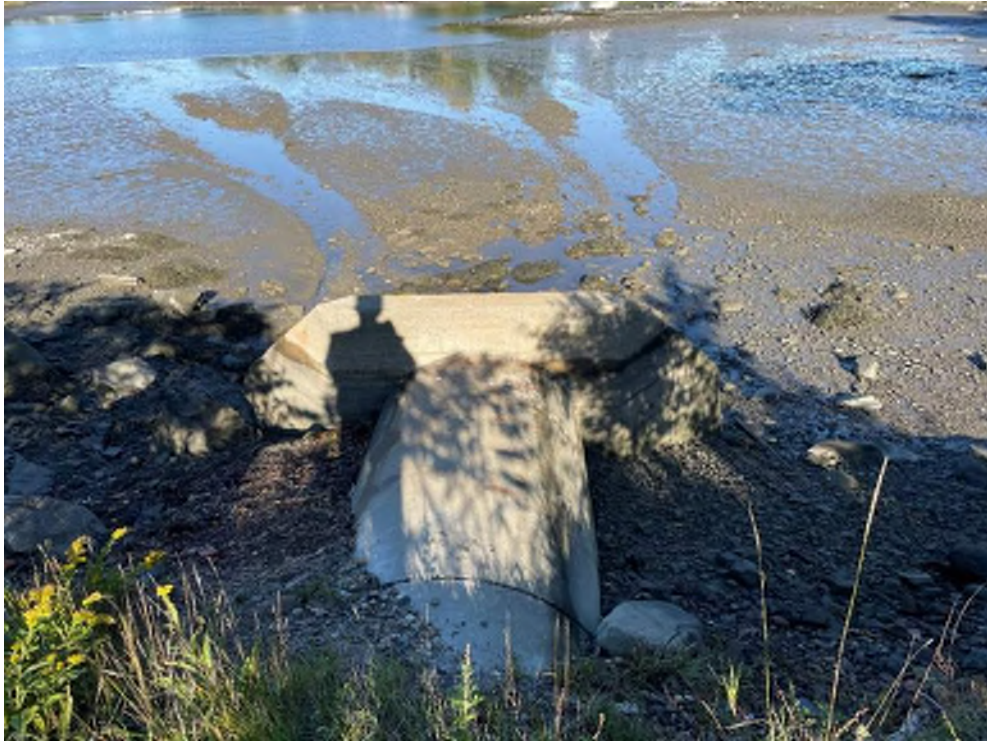
Photo 5 – Existing outfall headwall and exposed 48” RCP pipe looking northwest at approximate low tide. Taken 9/29/22
