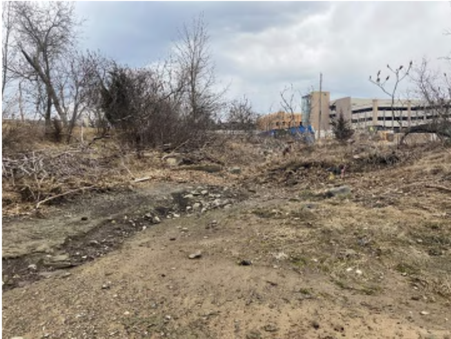
Photo 14 – Eroded channel in mitigation area at outlet of drainage swale (to be eliminated), looking south at approximate low tide. Taken 3/20/24
